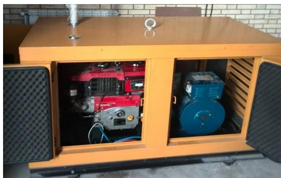
Figure 2- A general view of diesel generator
