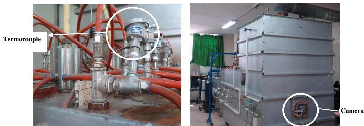
Figure 9- Exhaust Gas Stack and Quench Cooler
