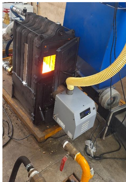
Figure 9- Burner & Boiler startup
