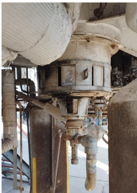
Figure 2- The real view of the main burner of furnace 204
